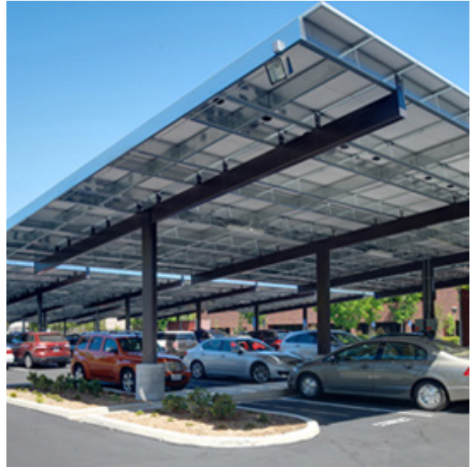
Solar canopies in surface parking lots.
