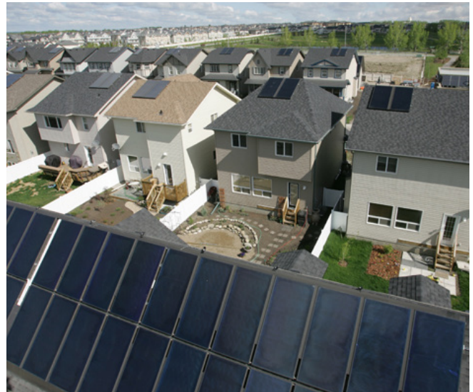
Solar panels on the roof of low-rise development.
