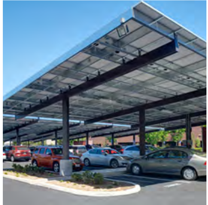
Solar canopies in surface parking lots.
