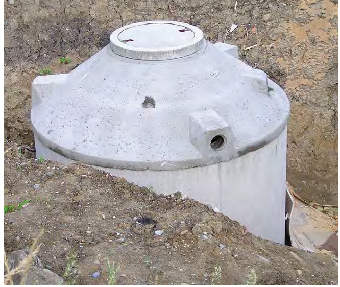
Collect, store, and distribute rainwater in underground storage tanks.
